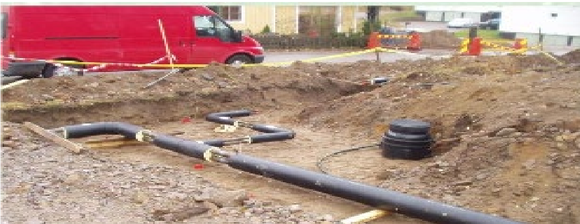
Figure 35 Twin pipes for a district heating network. [34]
