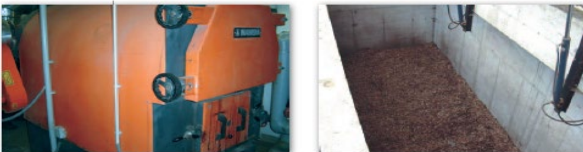
Figure 8 250kW medium size biomass boiler and storage bunker [10].
