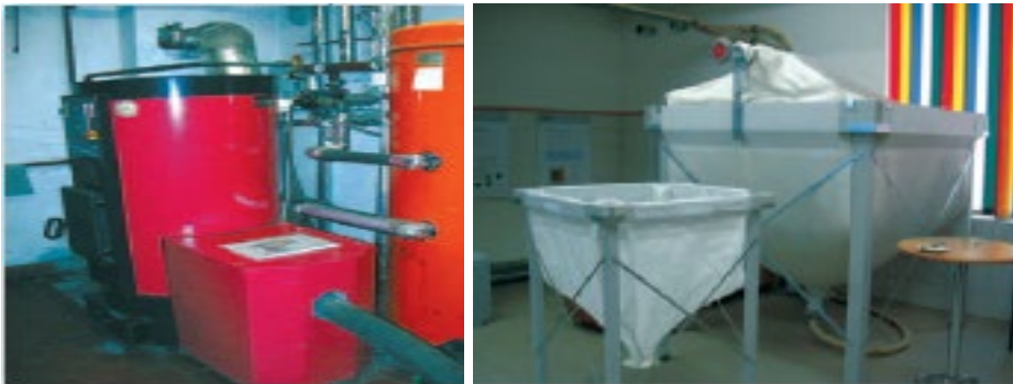
Figure 9 250kW biomass boiler for a single-family house and polypropylene silos for pellet (2-5t capacity) [10].
